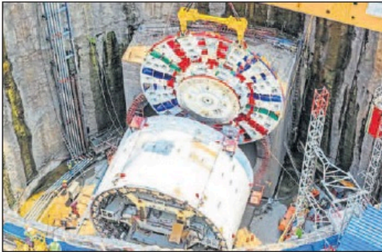
The machine, designed to excavate a large tunnel, is among the largest TBMs ever deployed for a railway project in India.
